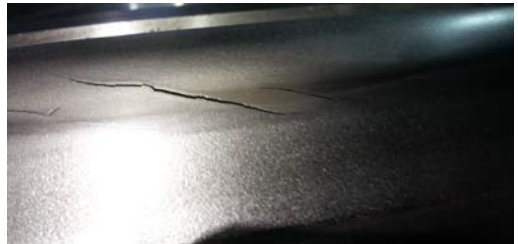
Fig. 5 Crack initialed at the surface of rails of derailment test facilities
