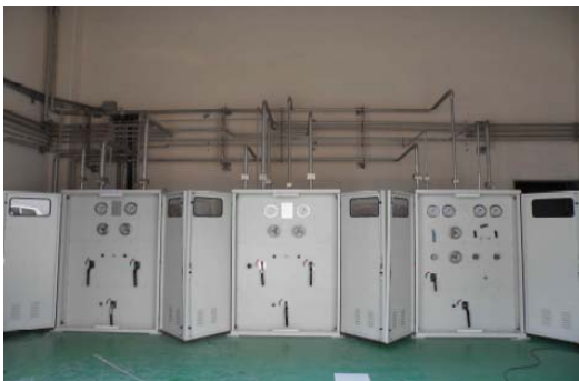
Fig. 4 From left side of photography, LOx, kerosene and NAS utility
