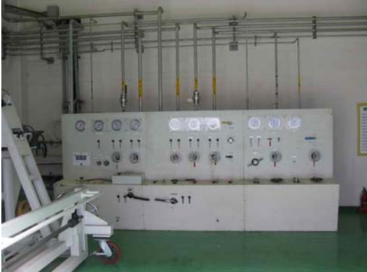
Fig. 2 Front side section of high pressure gas supply panel before modification of panels
