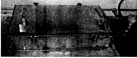
Fig. 2. Oil & Large Particle Strainer on the Top of Microfiltration Basin
