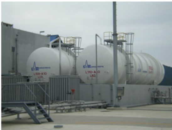
Fig. 1 Storage tanks for cryogenic liquid on launch complex
