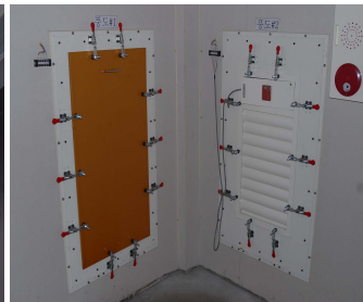
c) Smoke control damper
