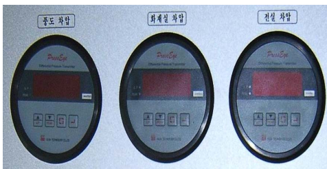
a) Pressure differential gauge
