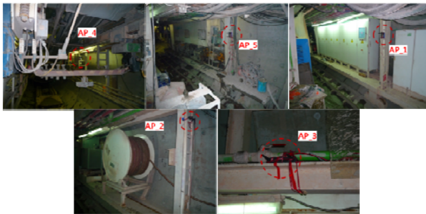
Figure. 12. Position of Installed APs (Boring Machine area)
