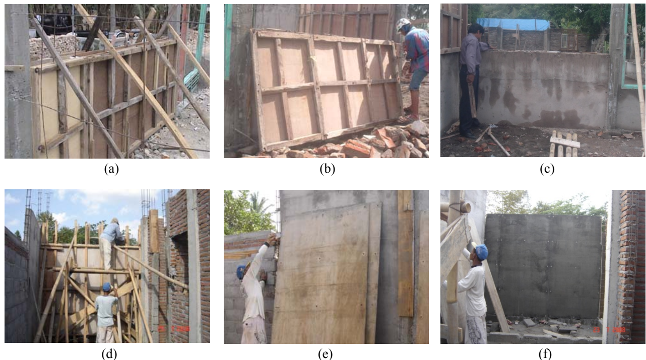
Figure 2. Old-CIP: (a) The Assembled Formwork, (b) The Dismantled Formwork, (c) The Constructed Wall; and New-CIP: (d) The Assembled Formwork, (e) The Dismantled Formwork, and (f) The Constructed Wall
