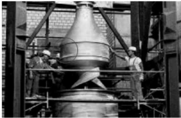
Fig. 10 The shaft casing of a CWP pump
