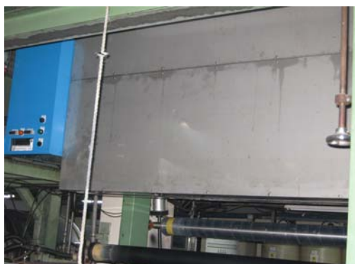
Fig. 3. Installed microwave generator in Kyung Il Dyeing Co.,LTD
