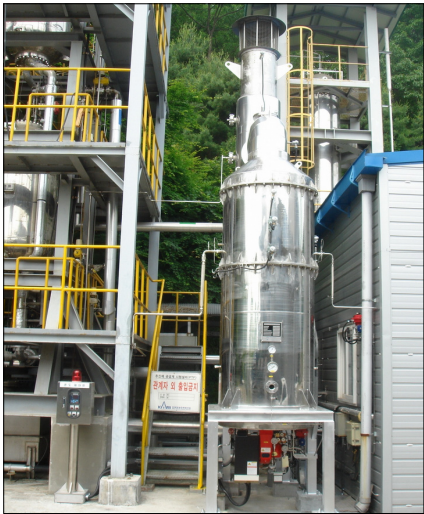
Fig. 3. The Photo. of Heating Apparatus
