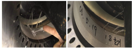
Fig. 6. Leak through adhesive Interface Failure
