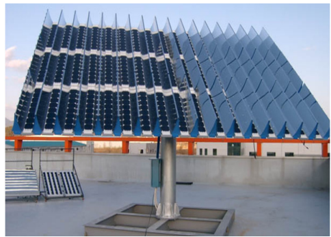
Fig. 5 Concentrator photovoltaic system
