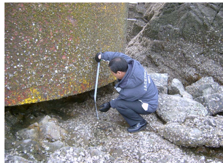
Fig. 3. Foundation scouring of a light beacon
