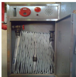
Fig. 1 Indoor hydrant system
