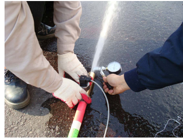
Fig. 4 Test of discharge pressure in hose reel hydrant system
