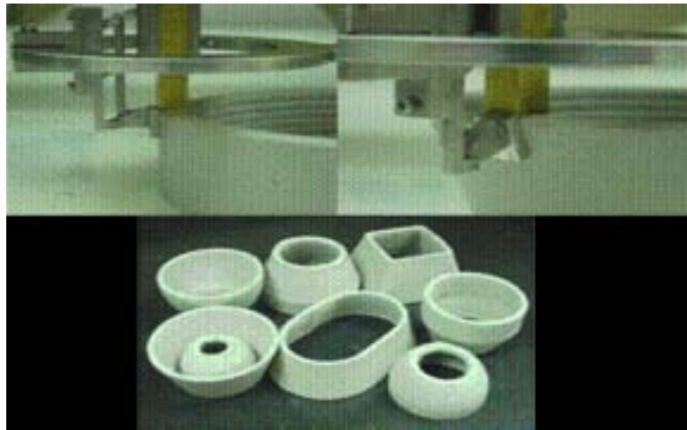
<Figure 11> CC process with the movable side trowel: (a) Actual process, and (b) various primitive geometries fabricated with the movable side trowel
