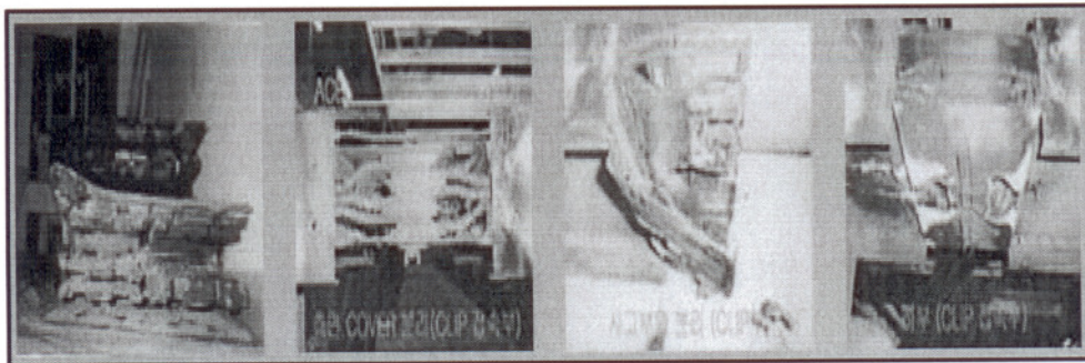
Fig. 2. A Case of Bus duct fire.
