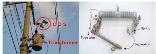
Fig. 1 Photograph of a cut out switch fuse hanging on an electric pole.
