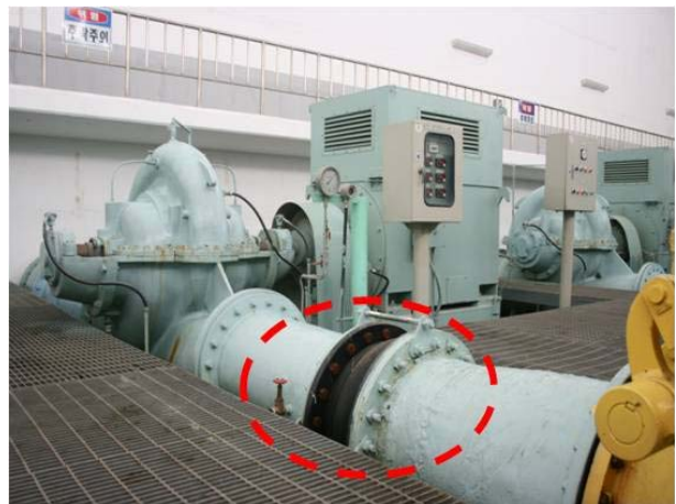
Fig. 3 Actually installed bellows location
