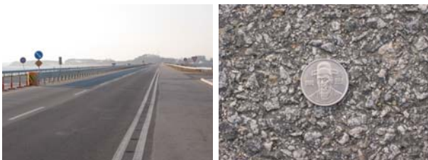
(a) A seawall at Seosan (b) Surface density Fig. 3 Information of test road
