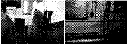
Fig. 4 Ventilation Facility and Oxygen Detection Device
