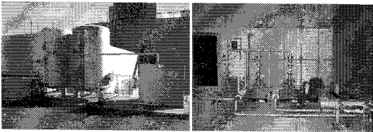
Fig. 5 Waste Water Disposal Facility
