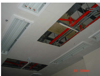
Figure 5. Mechanical equipment above the ceiling
