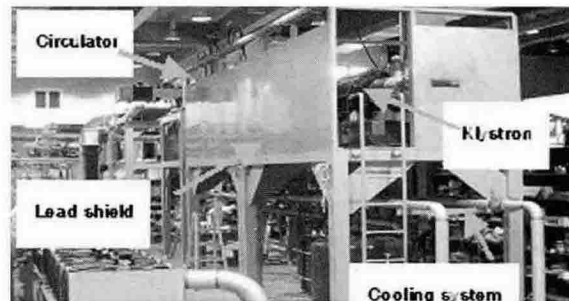
Figure 2. The installed HPRF system for 20MeV DTL
