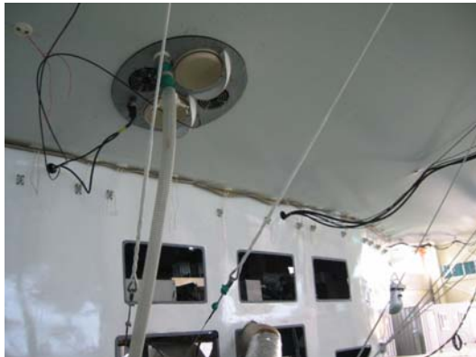
Fig. 10 Installation of a Pressure Control Unit
