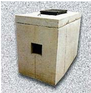
Fig. 3 A manhole for telecommunication
