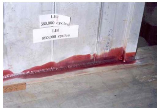
Fig. 7 Crack on the fillet joint of pocket plate
