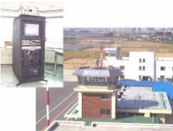
Fig. 6 Installed ground station at Ulsan airport
