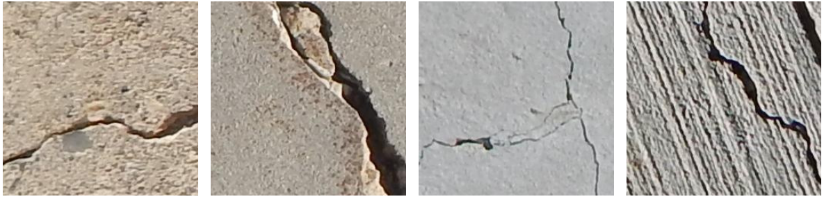
Fig. 1. Concrete crack images from USU
