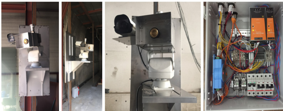
Fig. 5. Remote control fire extinguishing system for fire hose station
