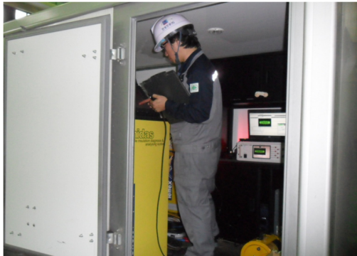
Fig. 3. AC high voltage test equipments.
