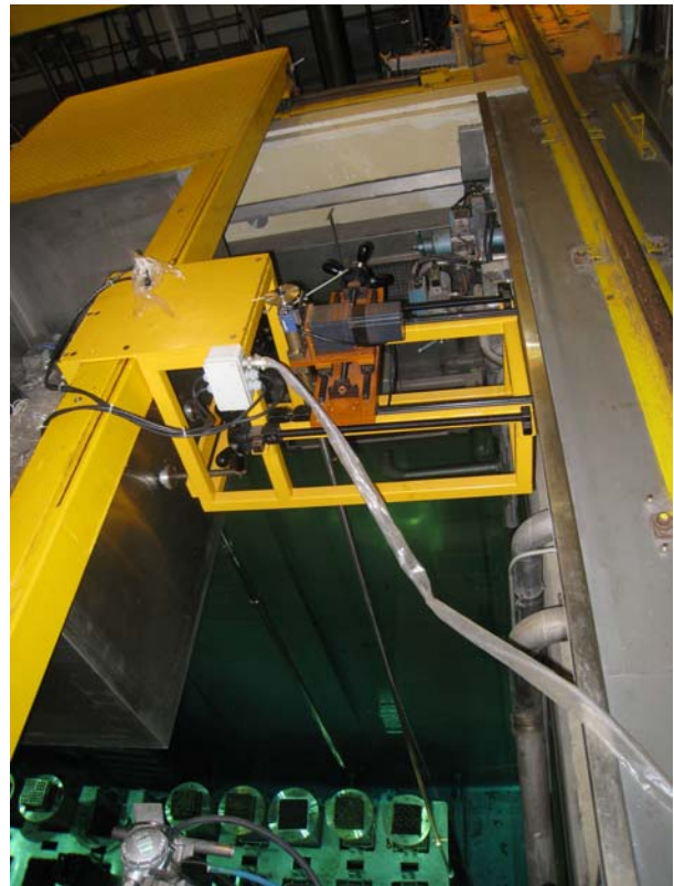
Fig. 1. Gamma-ray and neutron measurement system for spent fuel assembly at Korea Atomic Energy Research Institute.
