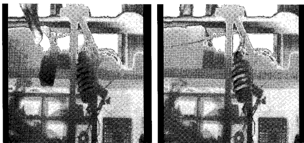
(a) Normal insulator (b) Faulty insulator
